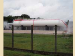
Water curtain systems
